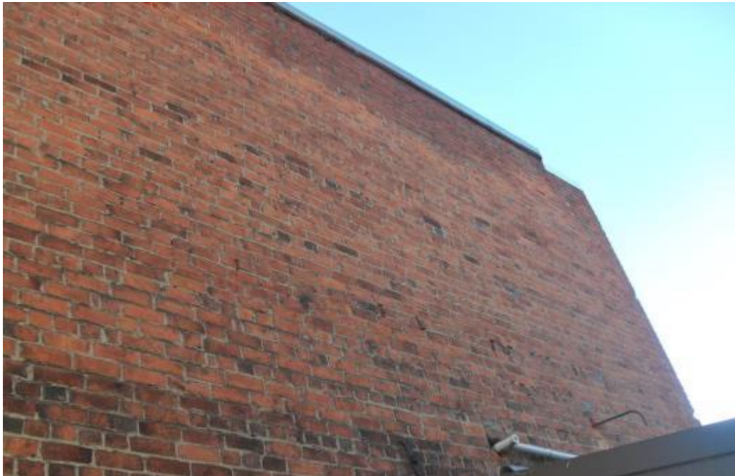
Figure 7 Damaged external URM wall
