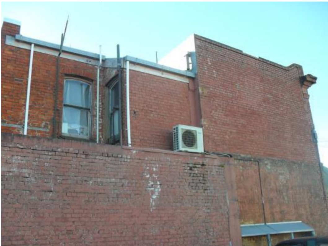
Figure 8 Damaged URM wall, various changes in shape of structure
