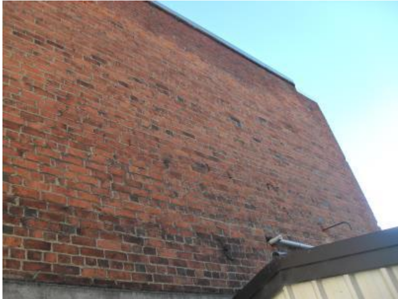
Figure 2 URM wall – No ties at floor or roof level
