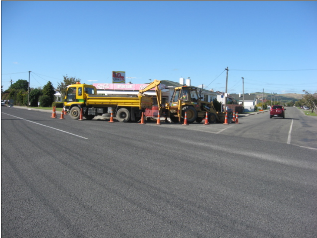
Downer Edi Works newly acquired JCB backhoe excavating a replacement pram crossing.
