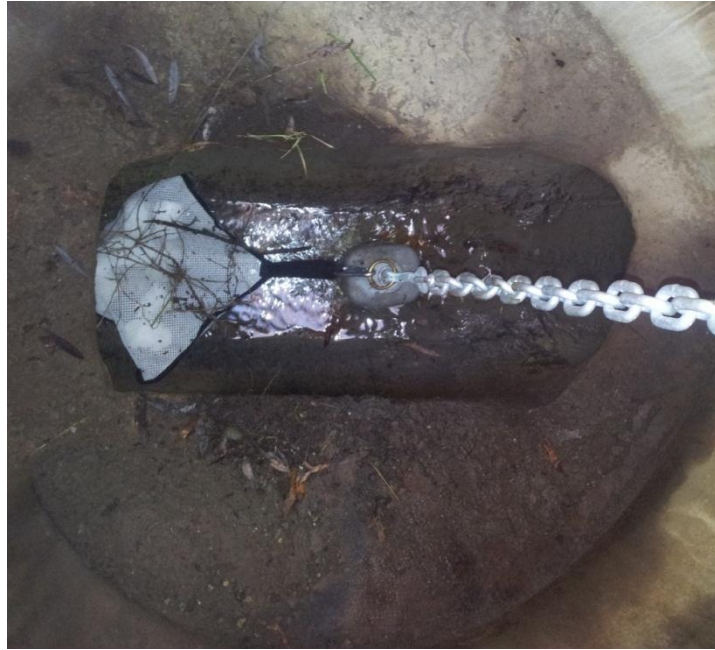
Passive skimmer filter bag inside manhole in South Gore industrial area
