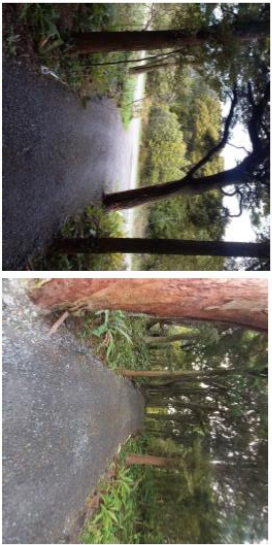
Job at Otara which used this system in close proximity to trees
