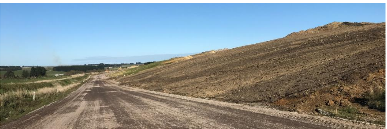
View of existing 20m high overburden mound taken from eastern haul road within site prior to grass growth
