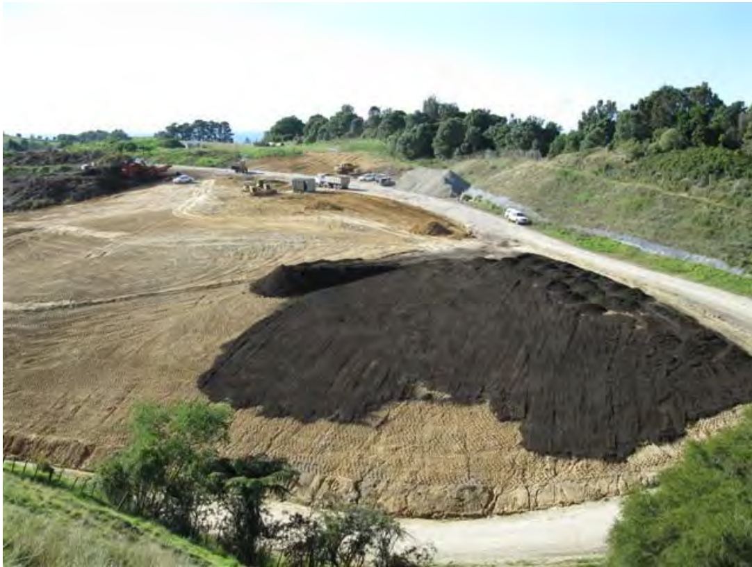
Photo 1: Spreading green waste mulch on the clay capping at Burma Road landfill 2011. Batter on front face is 3;1.
